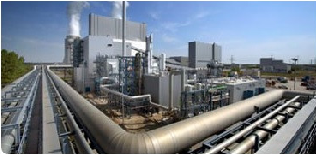
Picture of the Oxyfuel pilot plant in Schwarze Pumpe - May 2008
